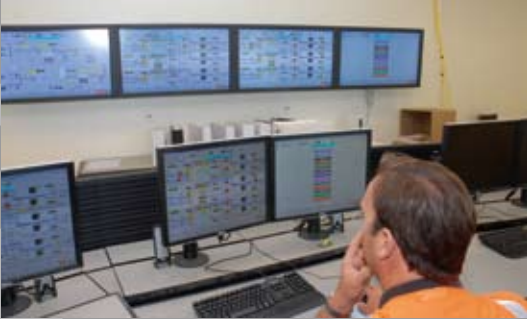
The system is monitored around the clock with a high-tech process control program. Photo: Orange County Water District.
